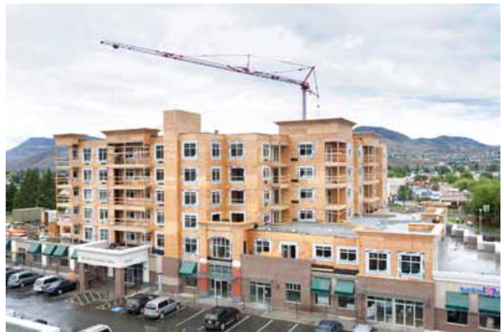
Five-storey wood-frame construction in Library Square in Kamloops, BC. Photo credit: Stephanie Tracey @ Photography West c/o WoodWORKS! BC
